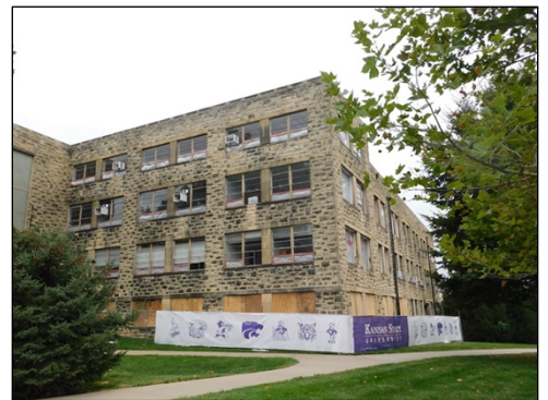
Both photos show demolition in progress of the Ahearn Gymnasium in Sept. 2023.
