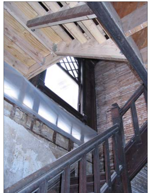
Looking up above the historic staircase to the newly constructed and relocated steps to the third floor master suite.
