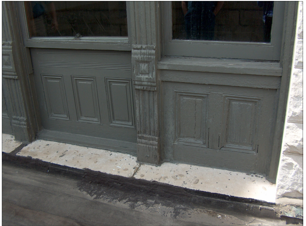
Deteriorated lead-based paint can create a health risk for building occupants.
